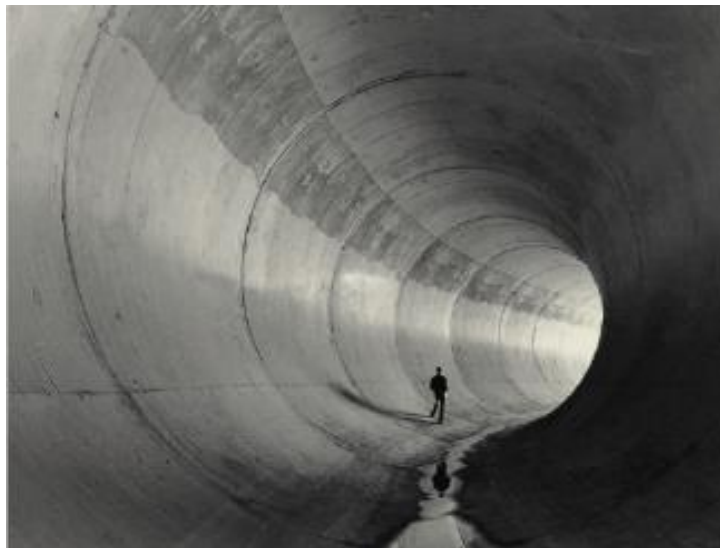
Figure 37: Columbia Basin Project's Soap Lake Siphon. http://www.nps.gov/history/history/online_books/dams/columbia_basin/sec2.htm
